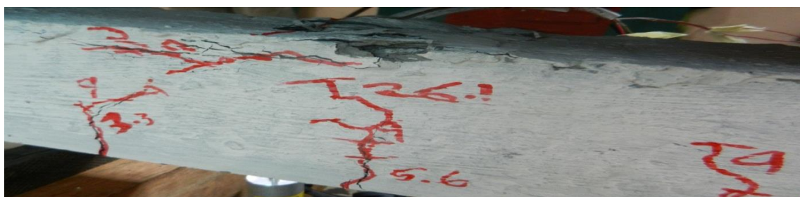
Fig. 12. Failure mode of control beam
