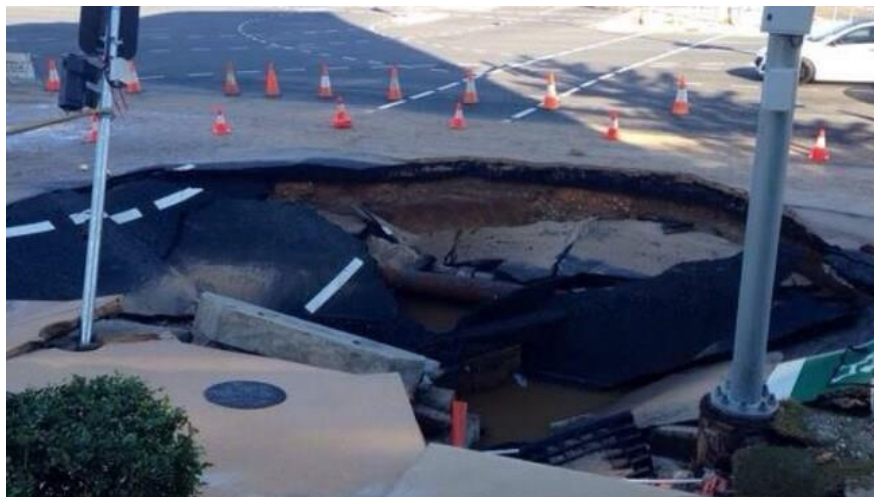
Figure 2.17. Sinkhole at Gold Coast Highway (Goldcoastbulletin, 2014)
