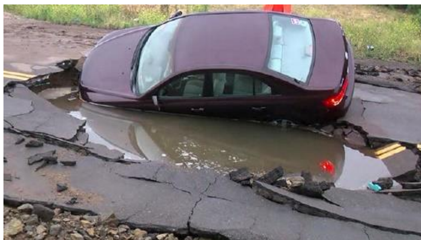
Figure 2.27. Car fallen into the sinkhole formed due to water pipe break (KGTV, 2017)
