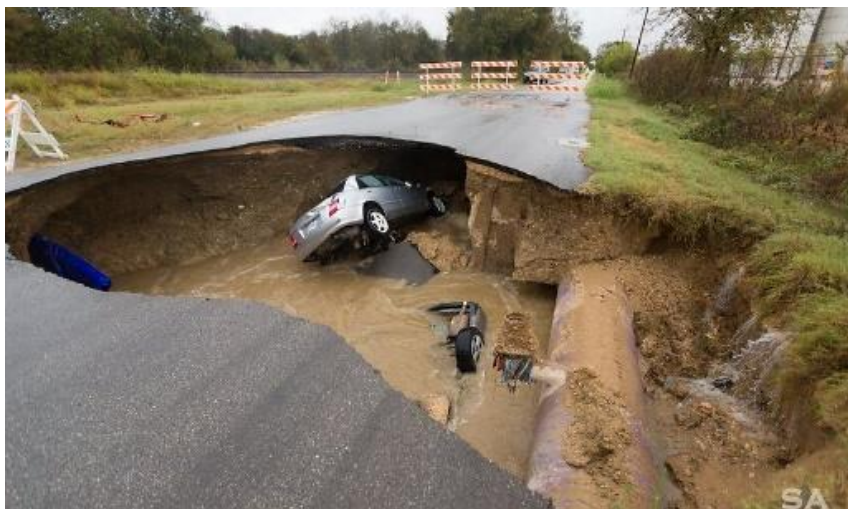
Figure 2.39. Sinkhole in Texas swallows two cars (Paulam, 2016)
