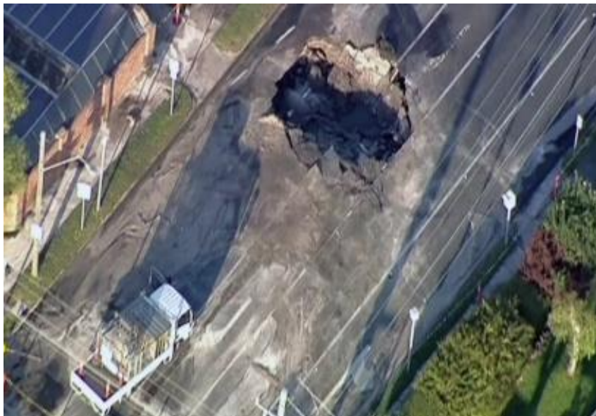
Figure 2.15. Massive sinkhole appeared in Glen Eira Road (Calligeros, 2015)
