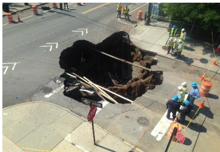
Figure 2.25. Sinkhole disrupts water supply (Berger, 2015)
