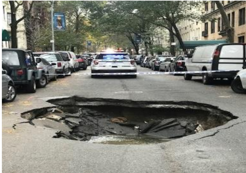
Figure 2.24. Sinkhole opened in the middle of a road (Business Insider, 2017)
