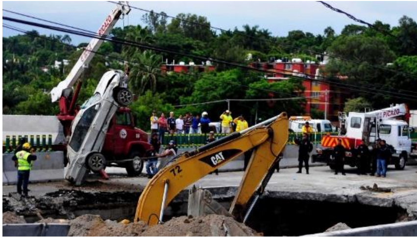
Figure 2.34. Sinkhole created due to a drainage leak (ABC News, 2017)
