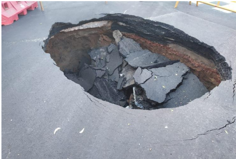
Figure 2.33. Sinkhole opened due to a leak in drainage pipe (The News Minute, 2019)
