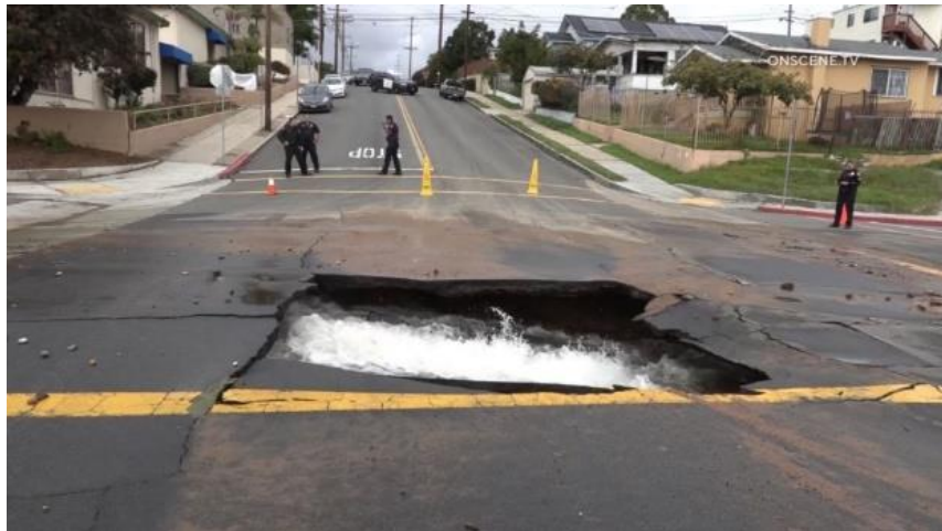
Figure 2.20. Sinkhole at a road in San Diego (McKinnon Broadcasting, 2020)
