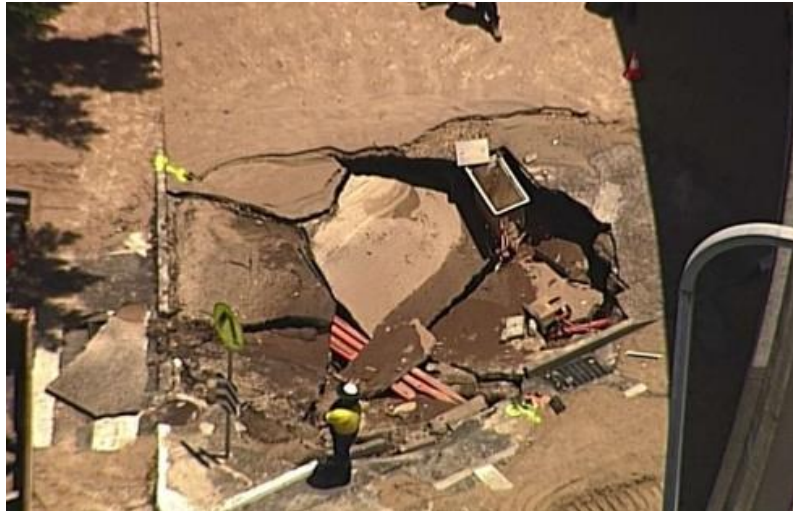
Figure 2.4. Sinkhole at Gold Coast due to water main leakage (ABC News, 2020)
