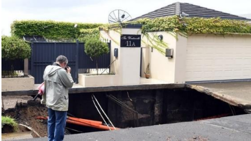
Figure 2.12. Sinkhole created due to line rupture (Levy, 2017)
