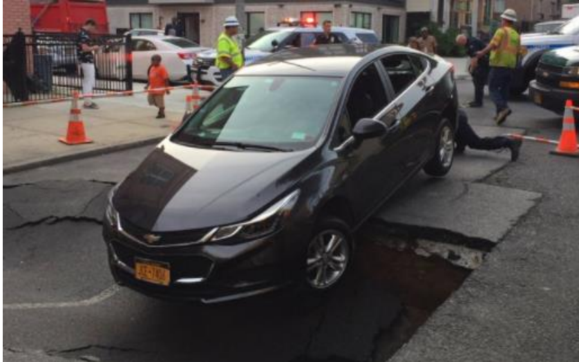
Figure 2.32. Sewer pipe break created a sinkhole in New York (Anon, 2019)
