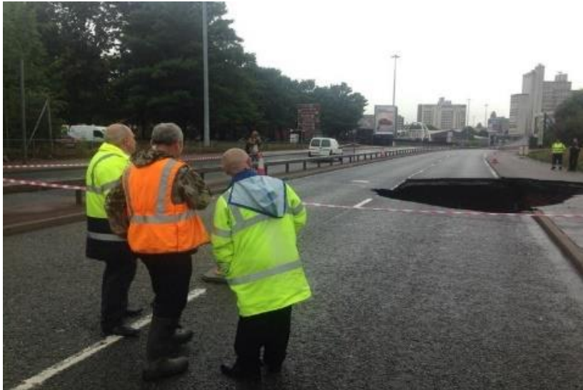
Figure 2.40. Sinkhole opened a second time in two months (The Guardian, 2015)
