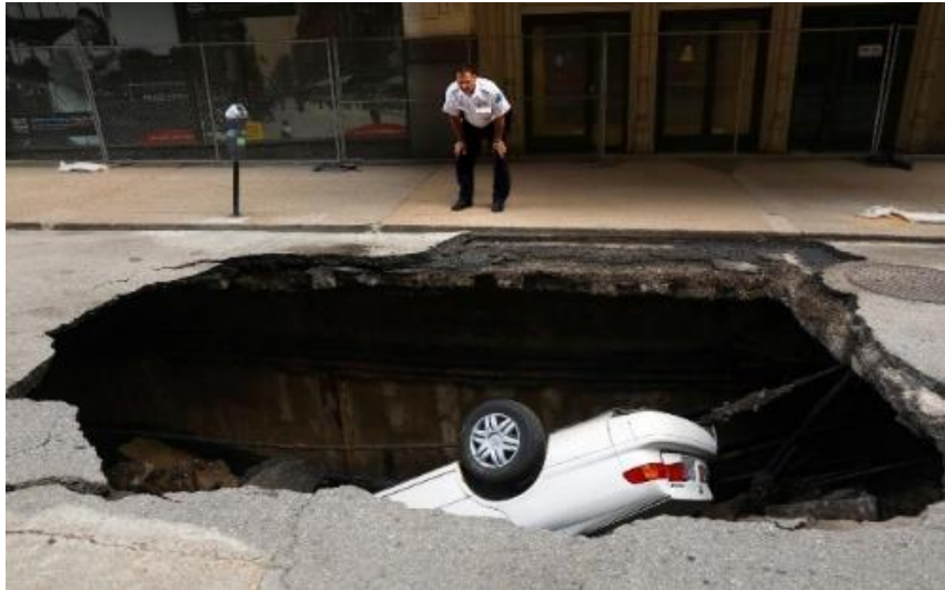
Figure 2.26. The gaping sinkhole ate a car (Morrison, 2017)
