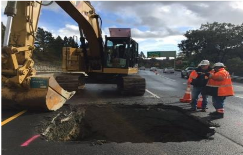
Figure 2.38. Broken drainage that caused the sinkhole (Detman, 2017)
