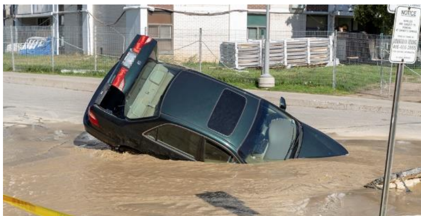
Figure 2.23. Car was swallowed by a sinkhole (toronto.citynews.ca, 2018)
