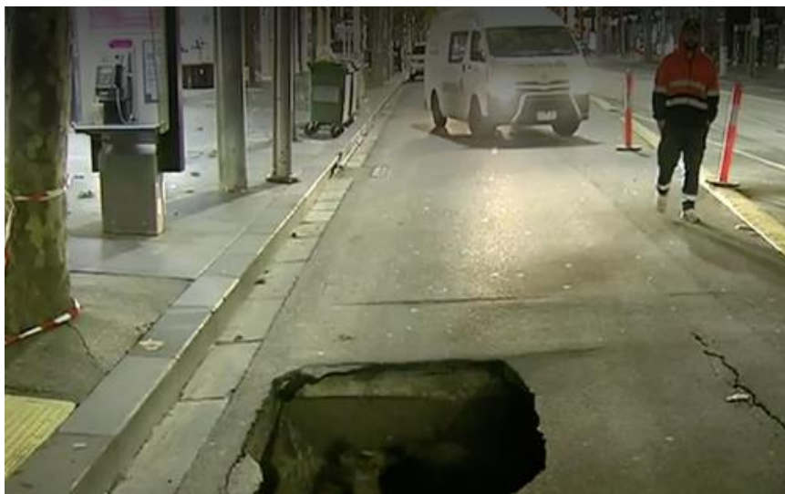
Figure 2.19. One-meter-wide sinkhole opened in Collin Street (Mimic News, 2020)
