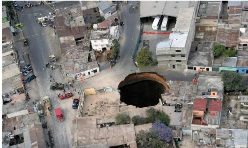
Figure 2.42. The sinkhole was opened due to a sewerage break (Avax News, 2007)
