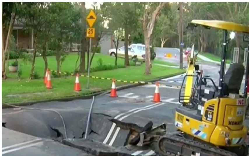
Figure 2.11. Sinkhole damaged a road in Mona Vale (Hit Network, 2017)
