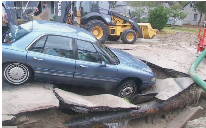
Figure 2.21. Sinkhole opened on a street in Norfolk (13newsnow.com, 2019)
