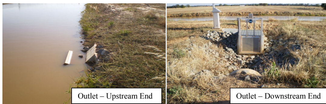
Figure 2.17 Undershot irrigation outlet
