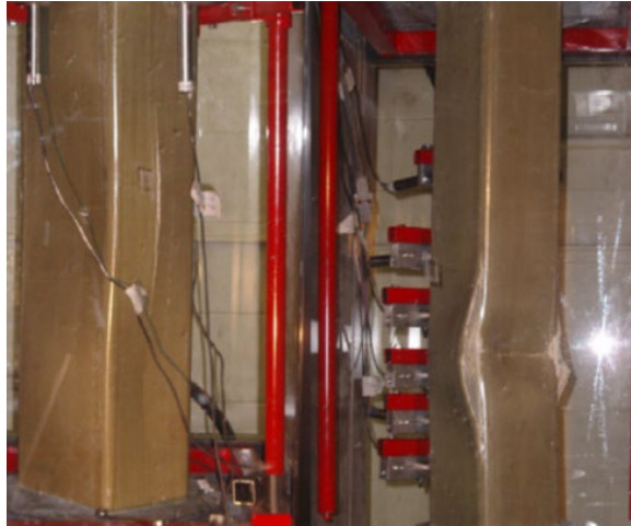
(a) Local buckling (Godat et al. 2013)
