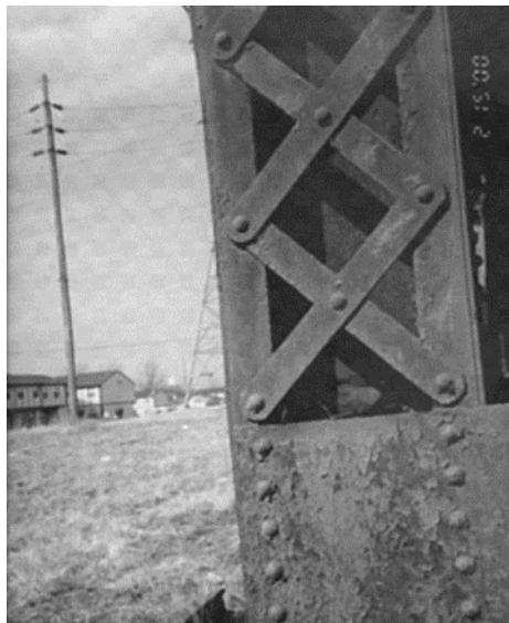
Figure 1.3 Corrosion of steel bridge column (Liu et al. 2005)
