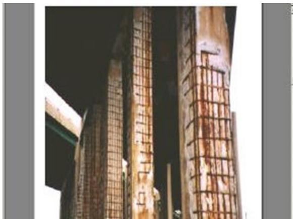
Figure 1.4 Steel corrosion of concrete columns
