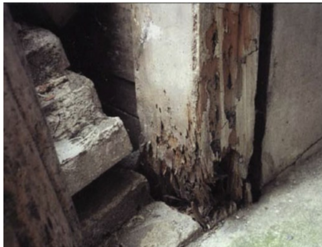
Figure 1.1 Timber column damage due to insects (Chang 2015)
