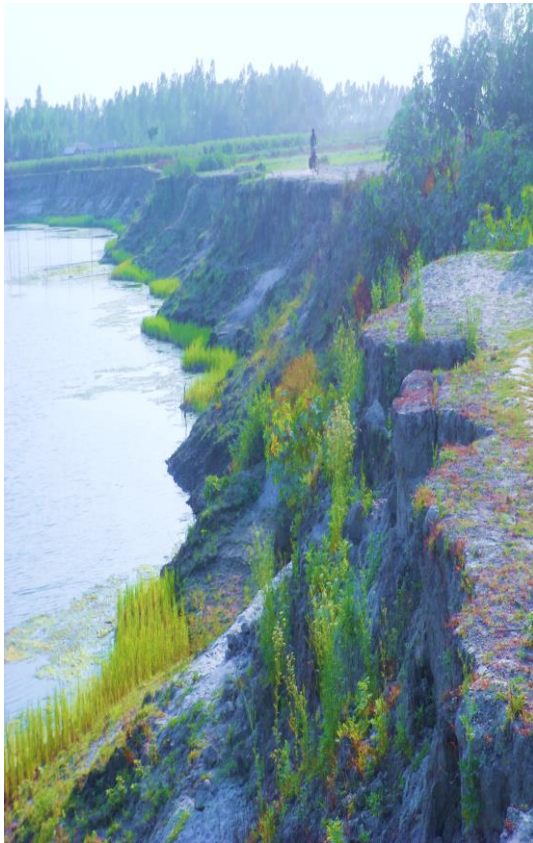
Riverbank erosion damage
