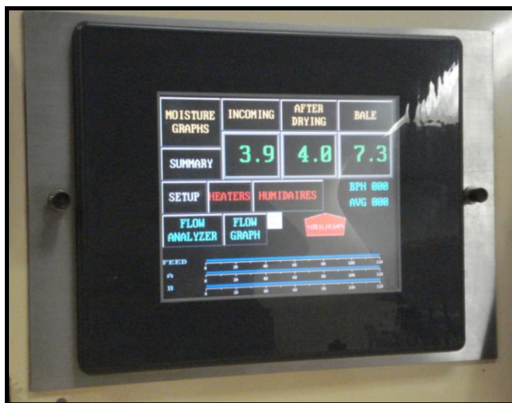
Figure 6.2: Terminal monitor in the control room
