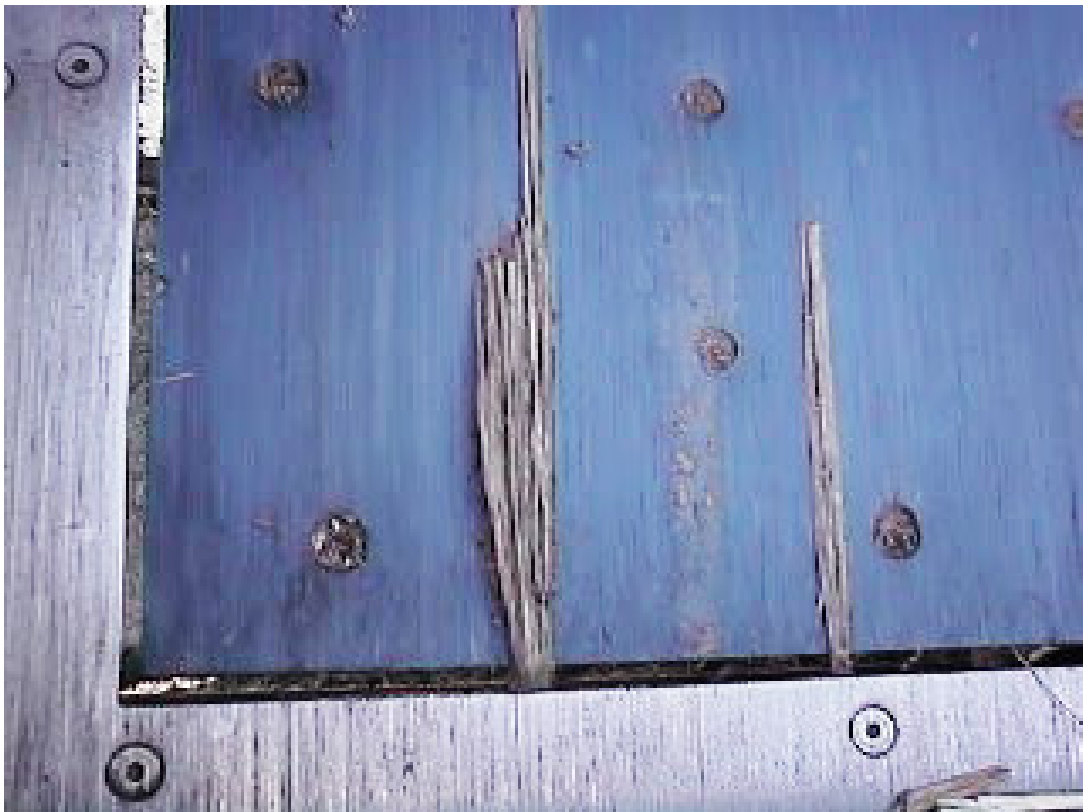
Figure 10-5. Leaf matter wedged between the weigh plate edge and the elevator floor.
