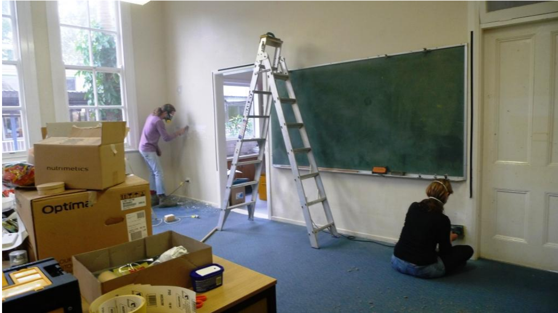
Figure 1.5: Parents worked to refurbish the old classroom during a school holiday break
