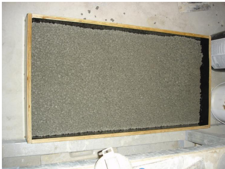
Figure 4.4 First layer of concrete being cast into 1000mm X 600mm X 100mm mould
