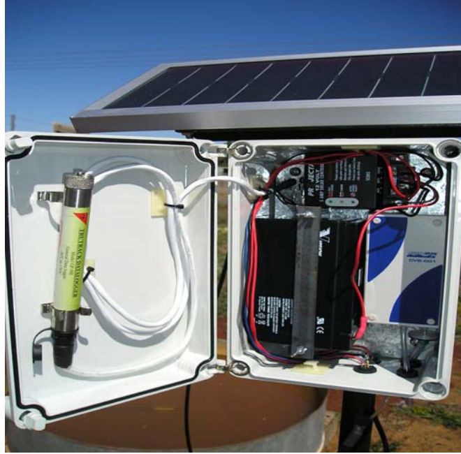
Figure 8 Datalogger, solar panel, battery, power management system and PST air breather system
