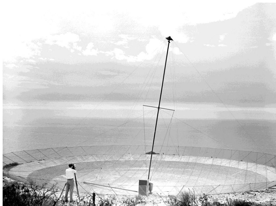
Figure 6.8. Upgrading the hole-in-the-ground telescope: (above) In February 1953 a concrete surface was added and the diameter extended from 22 to 24 m. The rotating wooden jig was used to position formwork for the concrete and also to finish the parabolic surface. (below) The completed dish showing the addition of the wire-mesh surface, the receiver mast, and the housing for the second stage of the receiver at the vertex. Gordon Stanley uses a theodolite to measure the angle of tilt of the mast. [courtesy: RAIA]
