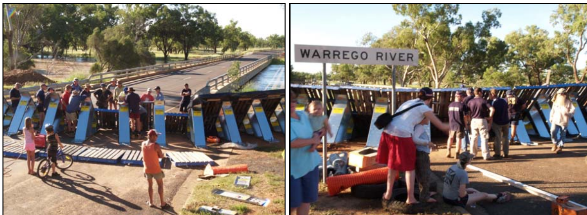
Figure 5.13. Some people in the community who helped during the construction of temporary levee during the 2008 flood in Charleville (Photo source: Chester Wilson)
