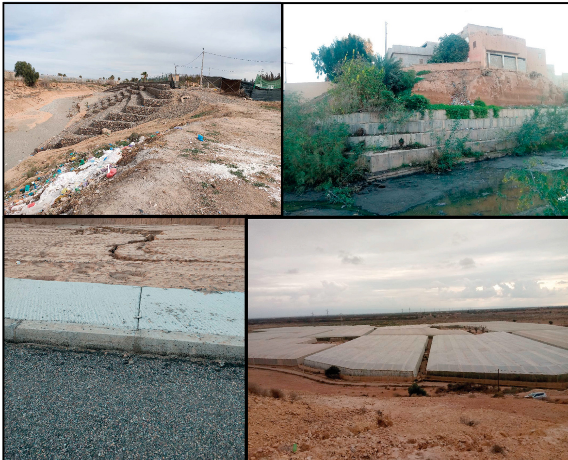
Fig. 13. Photos showing some solutions implemented to prevent the distribution of gully erosion in the study area.
