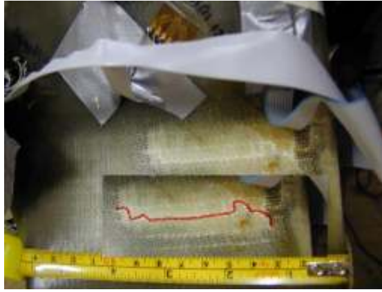
Figure 3 Early matrix failure and propagated crack and the at the blades root section.
