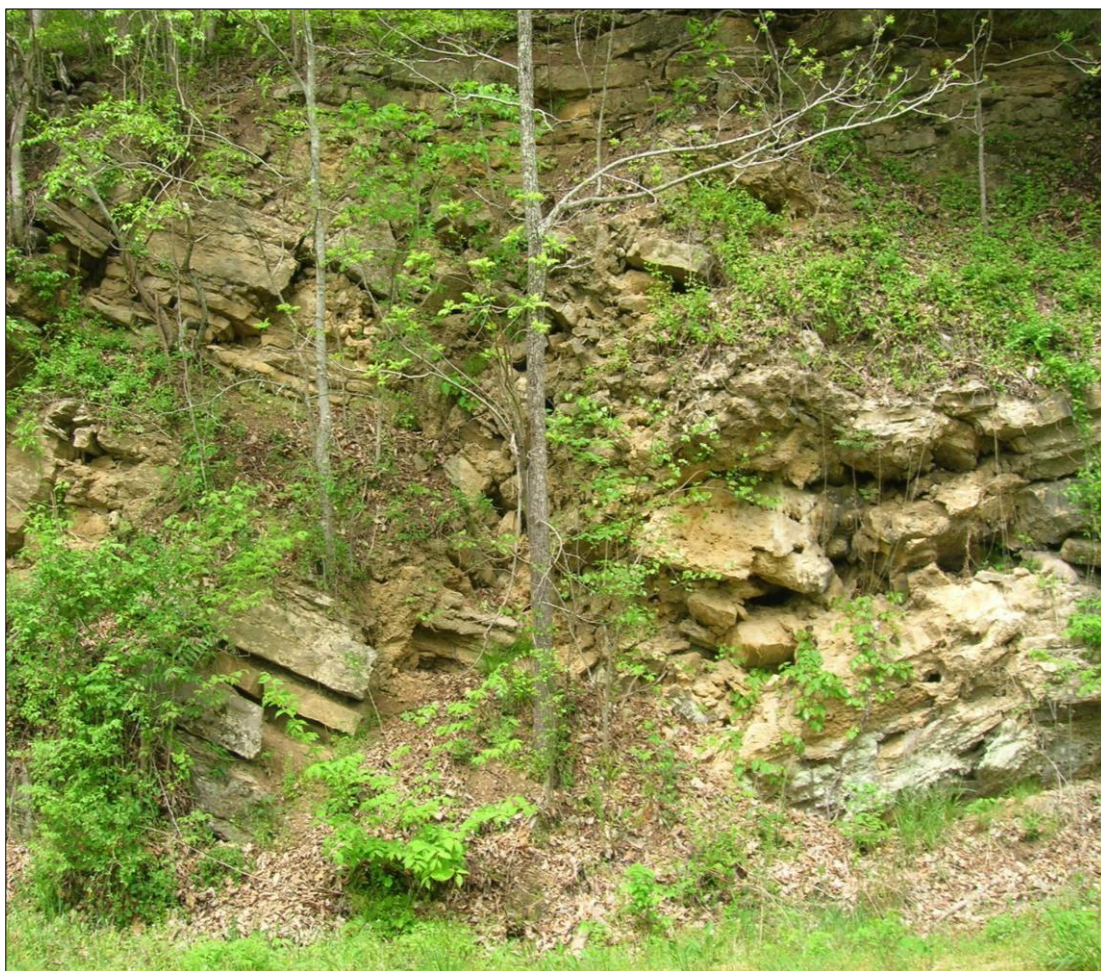
Figure 4.65 shows a collapsed cave on the side of Flynn Creek Road (photograph: Jana Ruth Ford).
