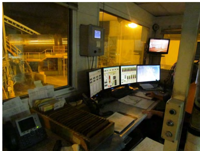
Figure: 4.11 The control room of the Eagle Farm Asphalt Plant
