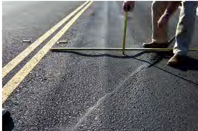
Figure: 1.1 Permanent deformation of asphalt mixture (Building-Science 2016)
