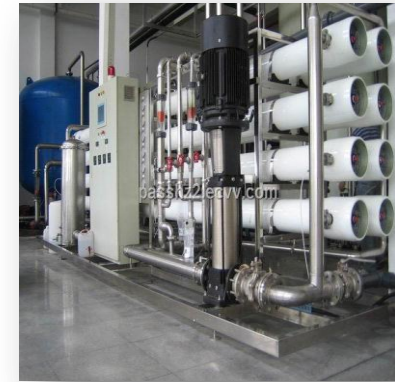
Membrane pre-treatment system
