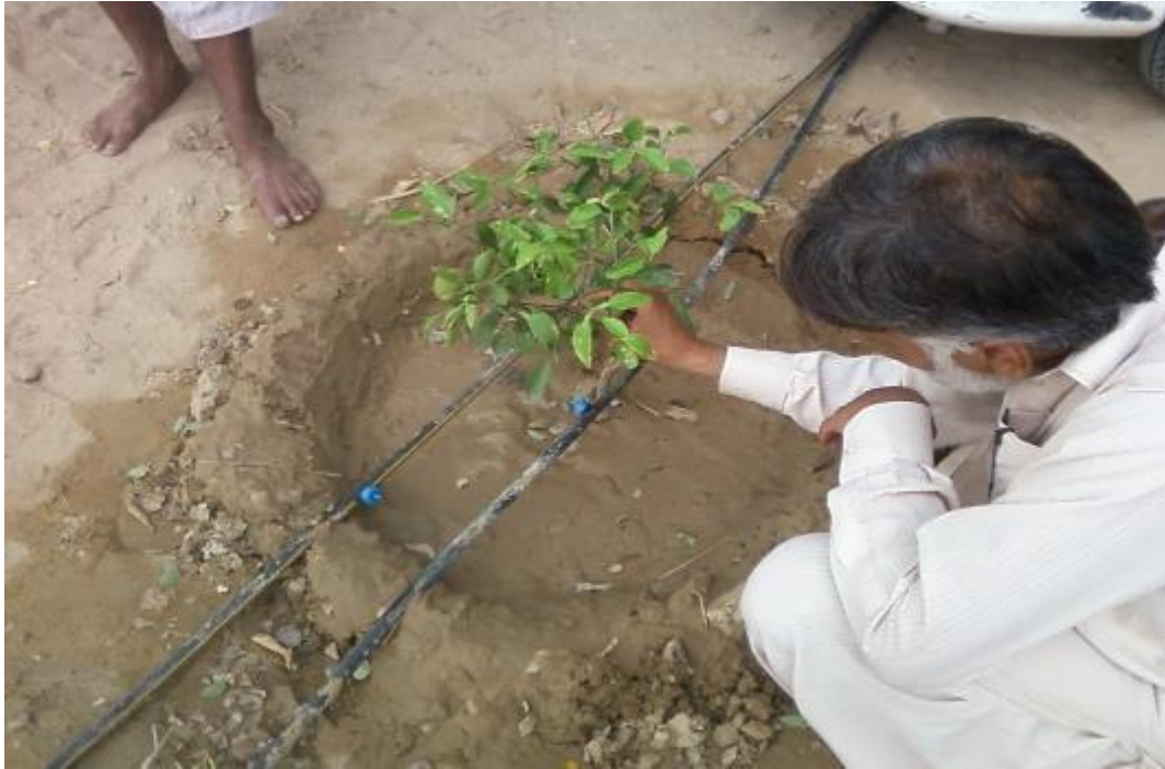
Figure 2.6: Close view of a drip irrigation system installed at another site in Punjab showing double drip tube along each plant row with button emitters (Akhtar, 2010).
