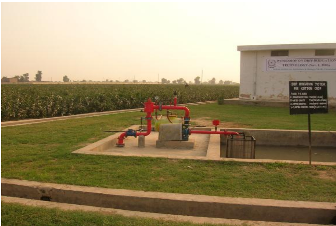
Figure 2.7: View of another pump shed, and water reservoir installed in Punjab region of Pakistan (Director General Agriculture, 2011).
