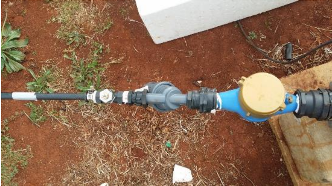
Figure 3.5: Multi-jet flowmeter and filter installed at the field test site.
