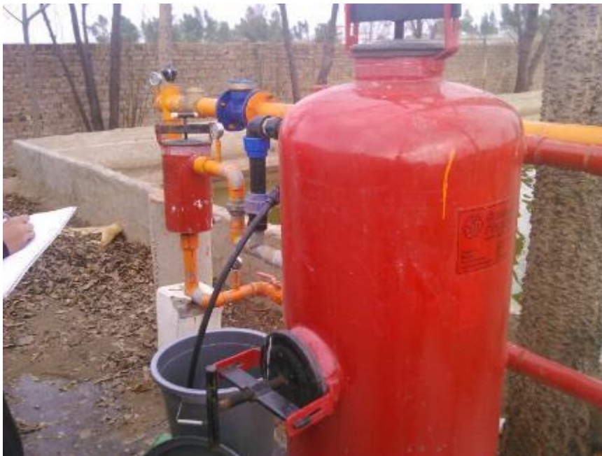
Figure 4.18: Disc and screen filter installed at pump shed.
