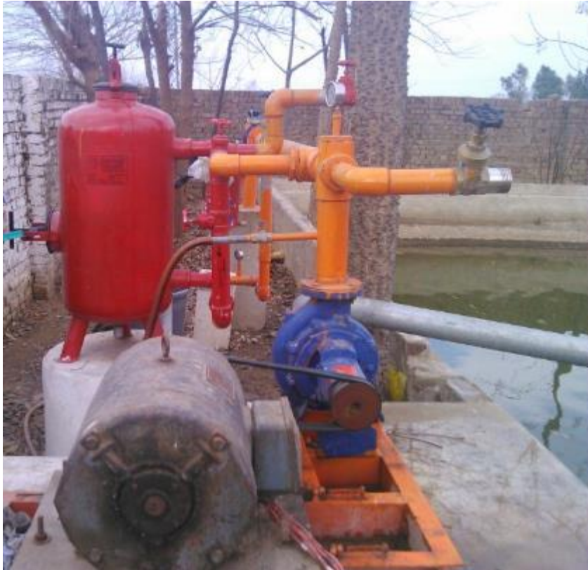
Figure 4.15: View of pump shed with filters installed along with pressure gauges and reservoir.
