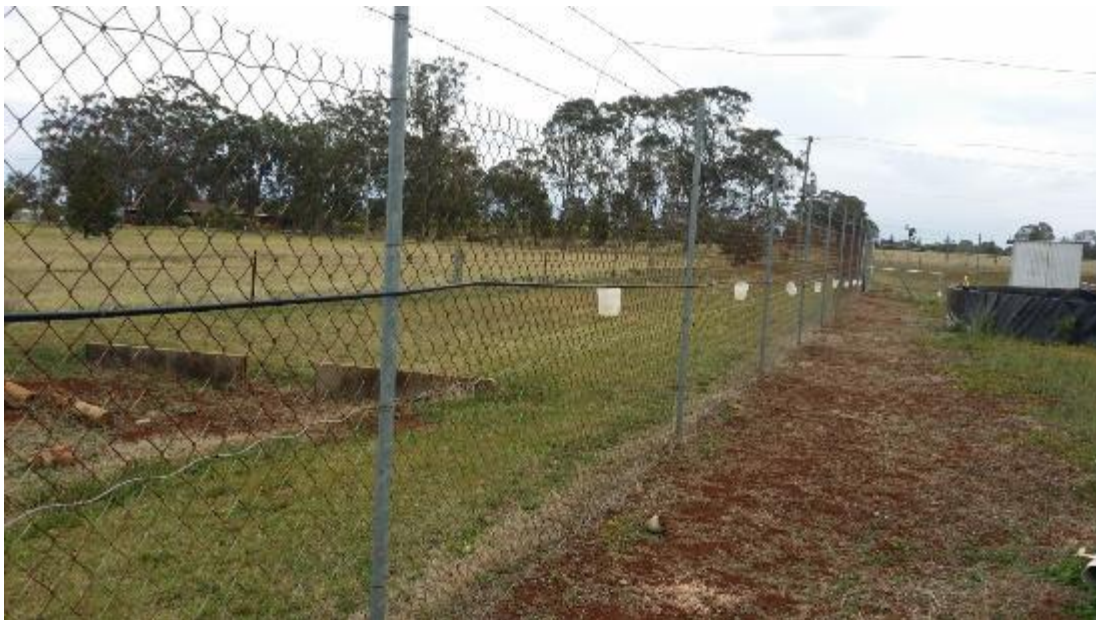
Figure 3.16: View of installed dripline on a downhill slope with water supply placed into the highest end of the dripline.
