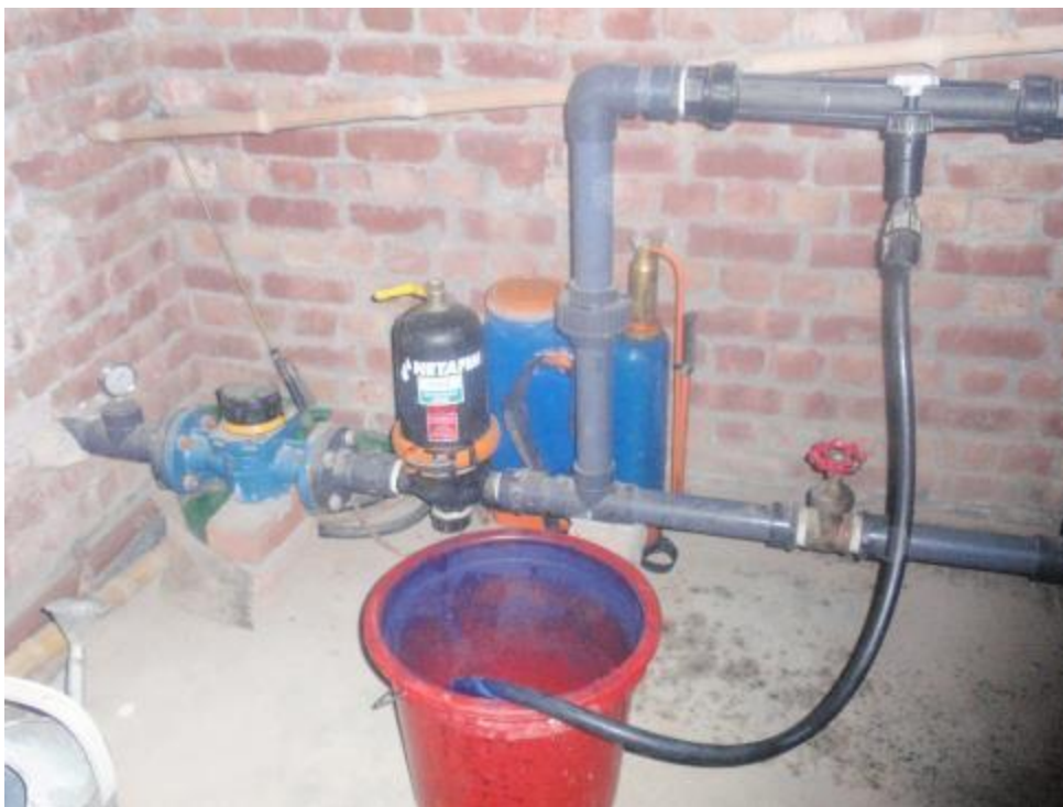
Figure 4.25: View of a screen filter installed at the pump shed along with venturi injector, flowmeter and pressure gauges.
