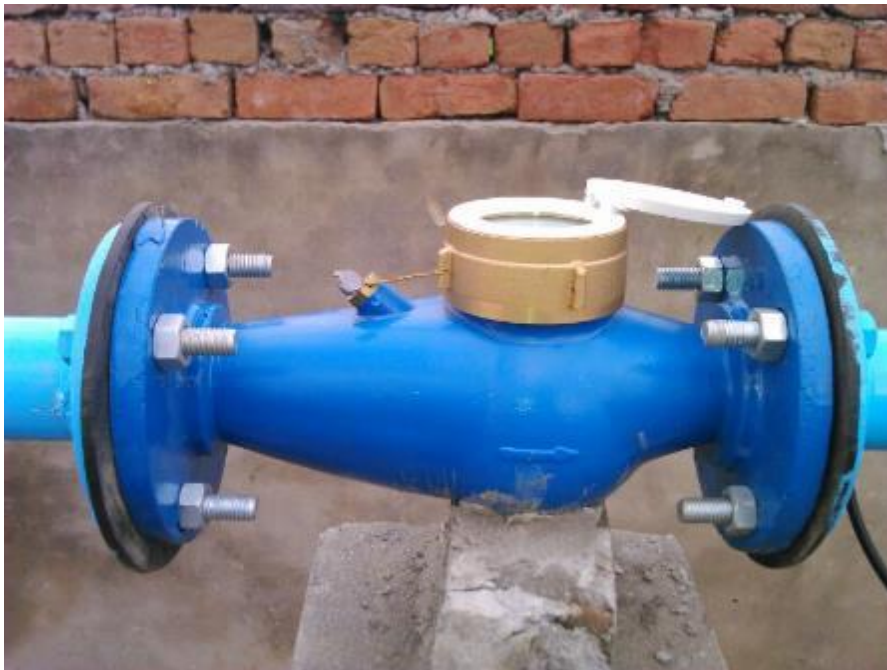
Figure 4.11: Close view of flow meter installed at the pump shed.
