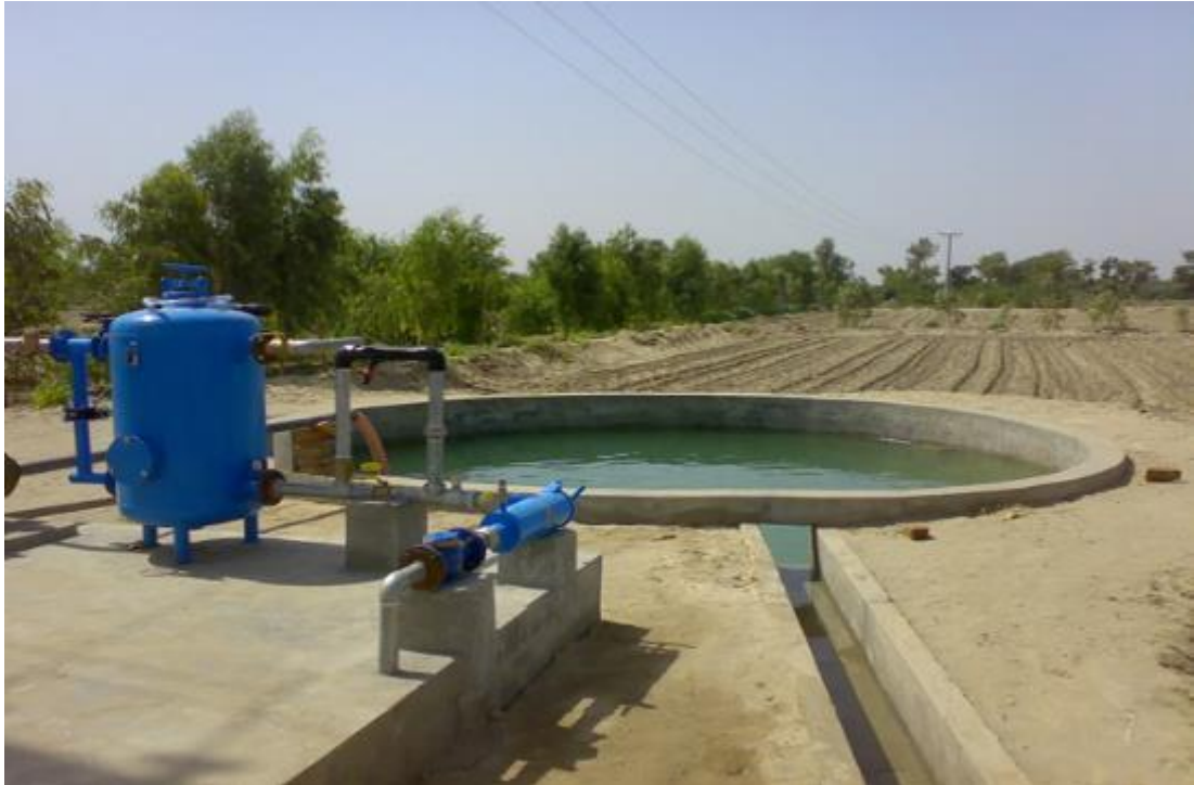
Figure 2.3: Pump shed installed at a drip irrigation site in Punjab, displaying the major components and water storage tank (Akhtar, 2010).
