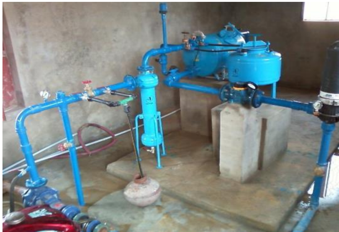
Figure 2.4: View of another pump shed installed in a closed room including filters and other major components (Akhtar, 2010).
