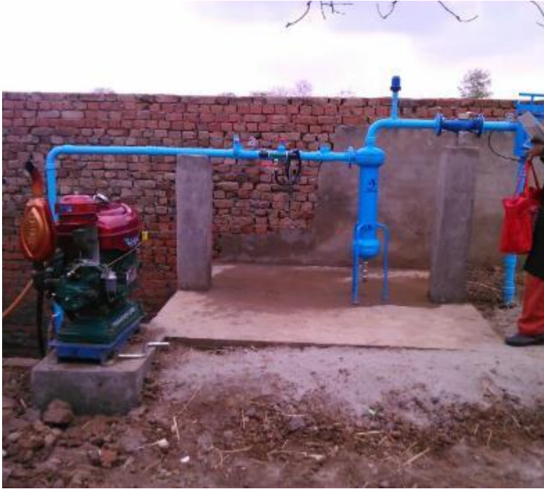
Figure 4.12: View of a pump shed with installed filters, flow meter, electric motor and venturi assembly.
