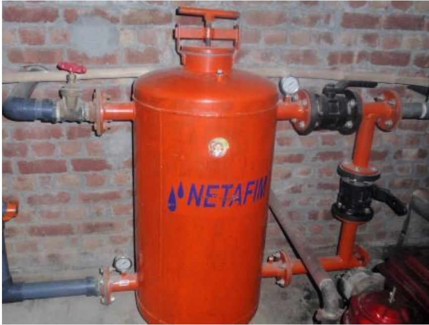
Figure 4.24: View of a disc filter installed at the pump shed.
