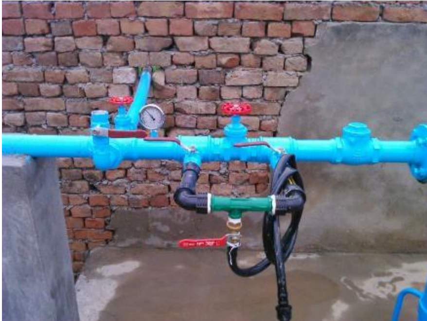
Figure 4.6: Pump shed showing installed venturi assembly and pressure gauges.
