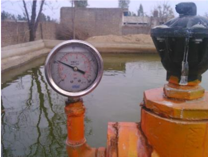
Figure 4.17: View of bourdon pressure gauge installed at pump shed.
