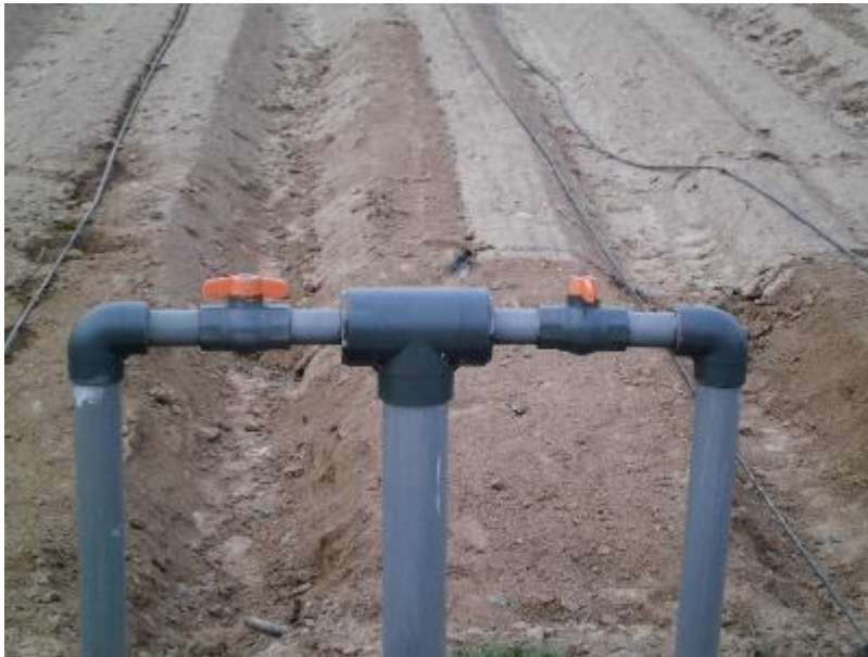
Figure 4.4: View of submain valve to operate the zone water flow.
