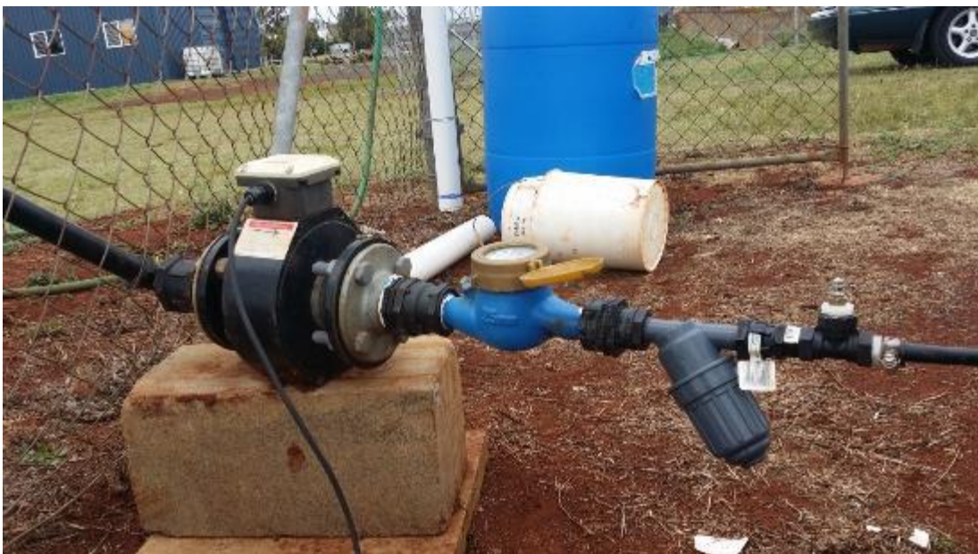
Figure 3.8: Water supply showing flowmeters, screen filter and the schrader valve installed at the field test
