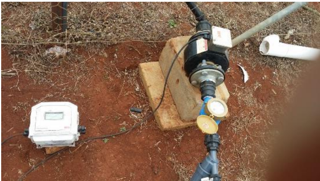
Figure 3.6: Electromagnetic (EM) flowmeter installed at the water supply point.
