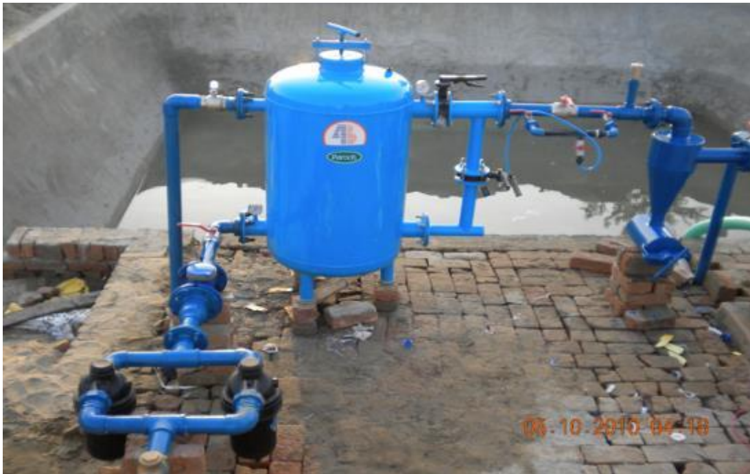
Figure 2.2: View of a pump shed installed, showing filters, venturi assembly, pressure gauges, flow meter and water reservoir (Akhtar, 2010).
