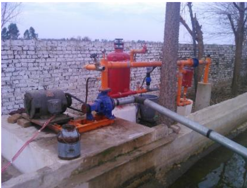
Figure 4.16: Back view of pump shed along with filters and reservoir.
