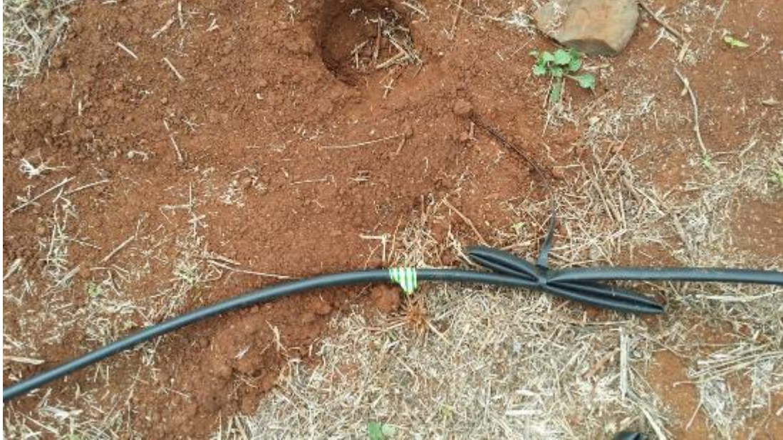
Figure 3.17: End of the dripline is blocked using plastic tie wires.
