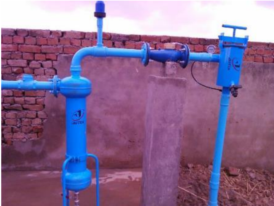
Figure 4.7: View of a screen filter, disc filter and flow meter installed at the pump shed.
