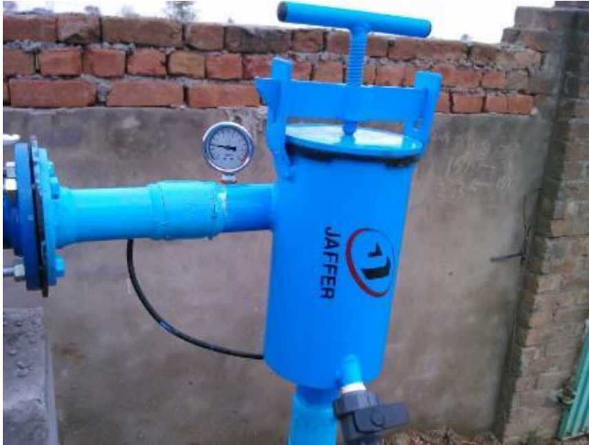
Figure 4.10: Screen media filter and pressure gauge installed at the pump shed.
