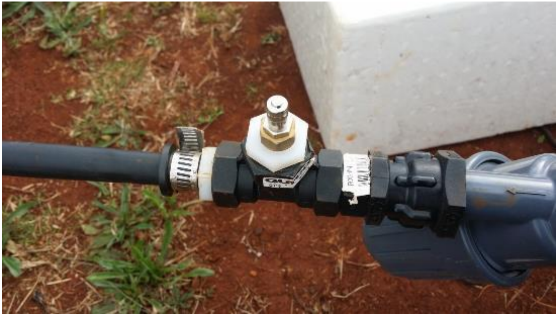
Figure 3.9: Close view of the schrader valve installed at the supply end of the dripline.
