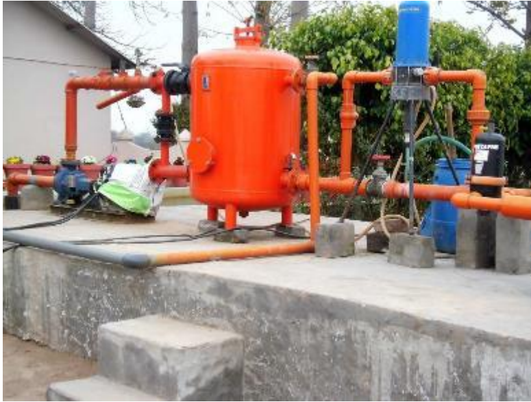
Figure 4.3: Pump shed including gravel filter, disc filter, flowmeter, venturi injector and pressure gauges installed on field.
