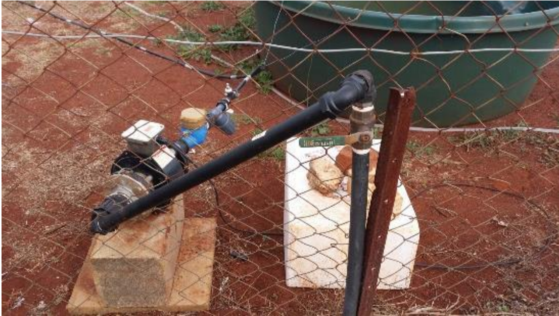
Figure 3.7: Back view of the water supply installed at the field test site.
