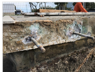
(b) Galvanic corrosion in pontoon decks (Image courtesy of CD Sorbello)
