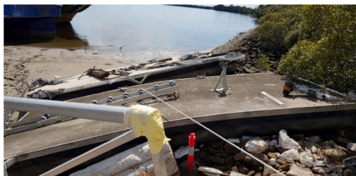
(a) Damaged pontoon during the 2022 Queensland flood (Image courtesy of CD Sorbello)
