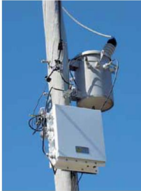
Figure 2.7: Low Voltage Regulator (LVR) mounted on a SWER transformer pole for 240V single phase supply [54].
