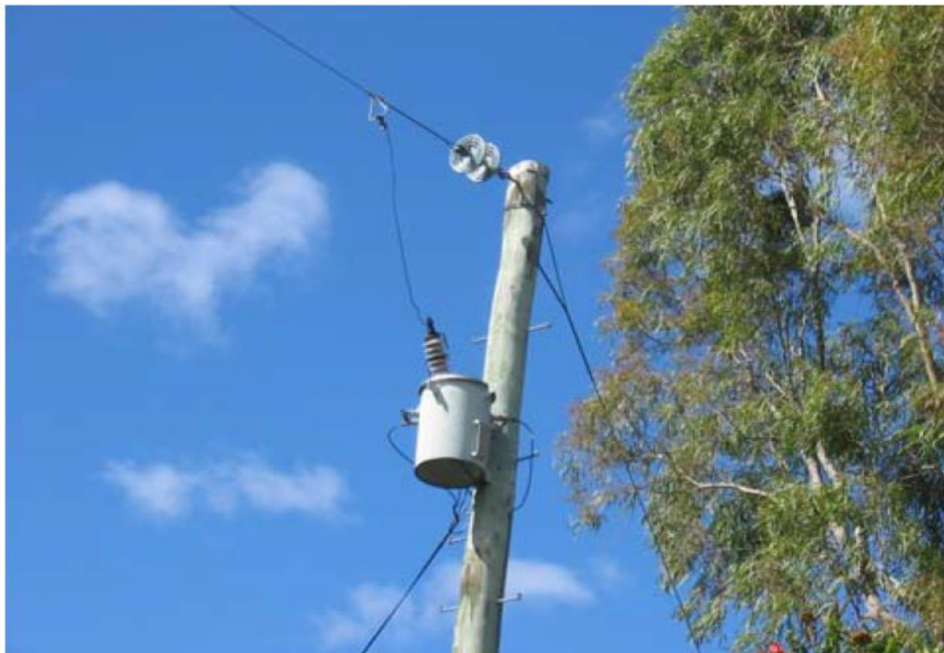
Figure 2.4: SWER customer transformer [34].
