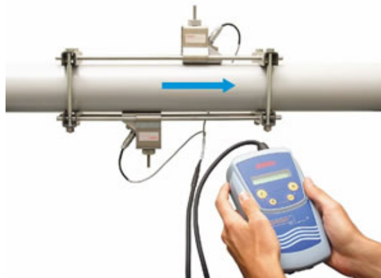
Figure 5 Portable ultrasonic flowmeter
