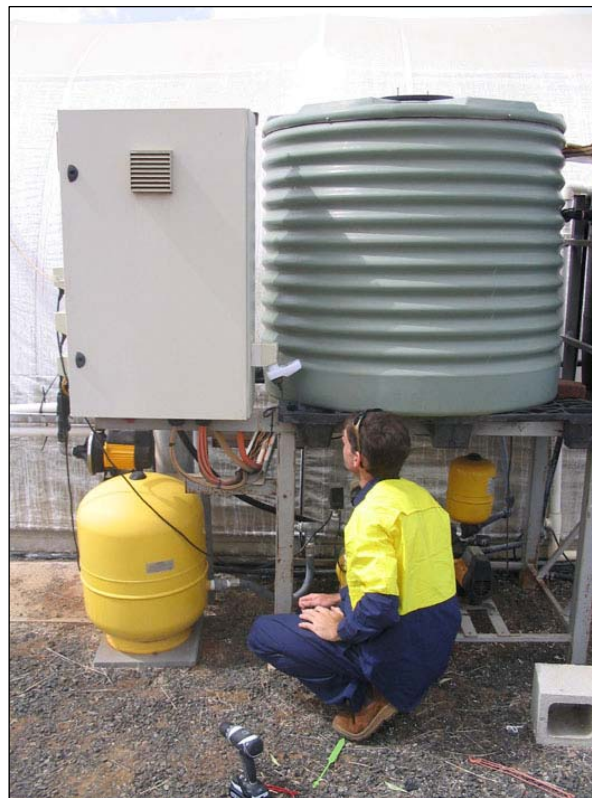
Testing the Hot water heater and small pump (Right)
