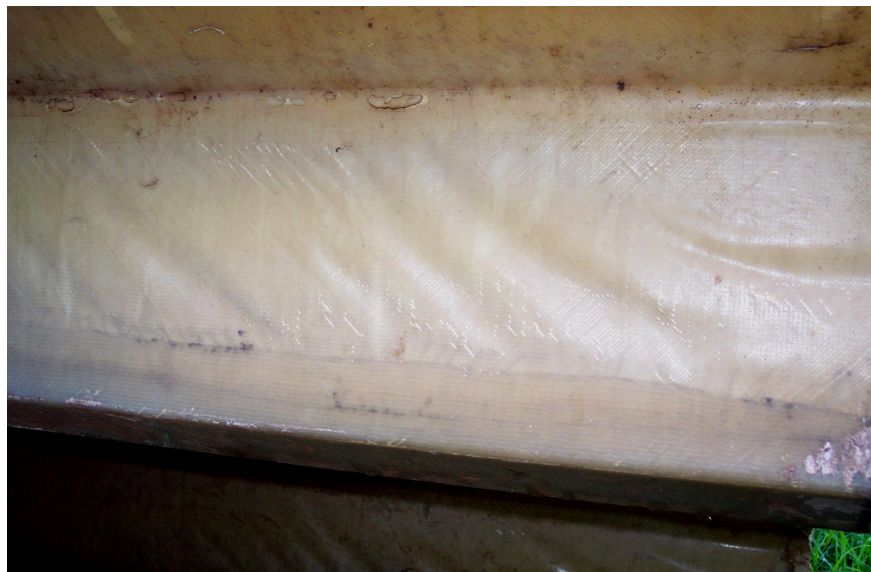
Figure 4.1 Distortions that appeared along the sides of the decking unit that were attributed to shrinkage forces.
