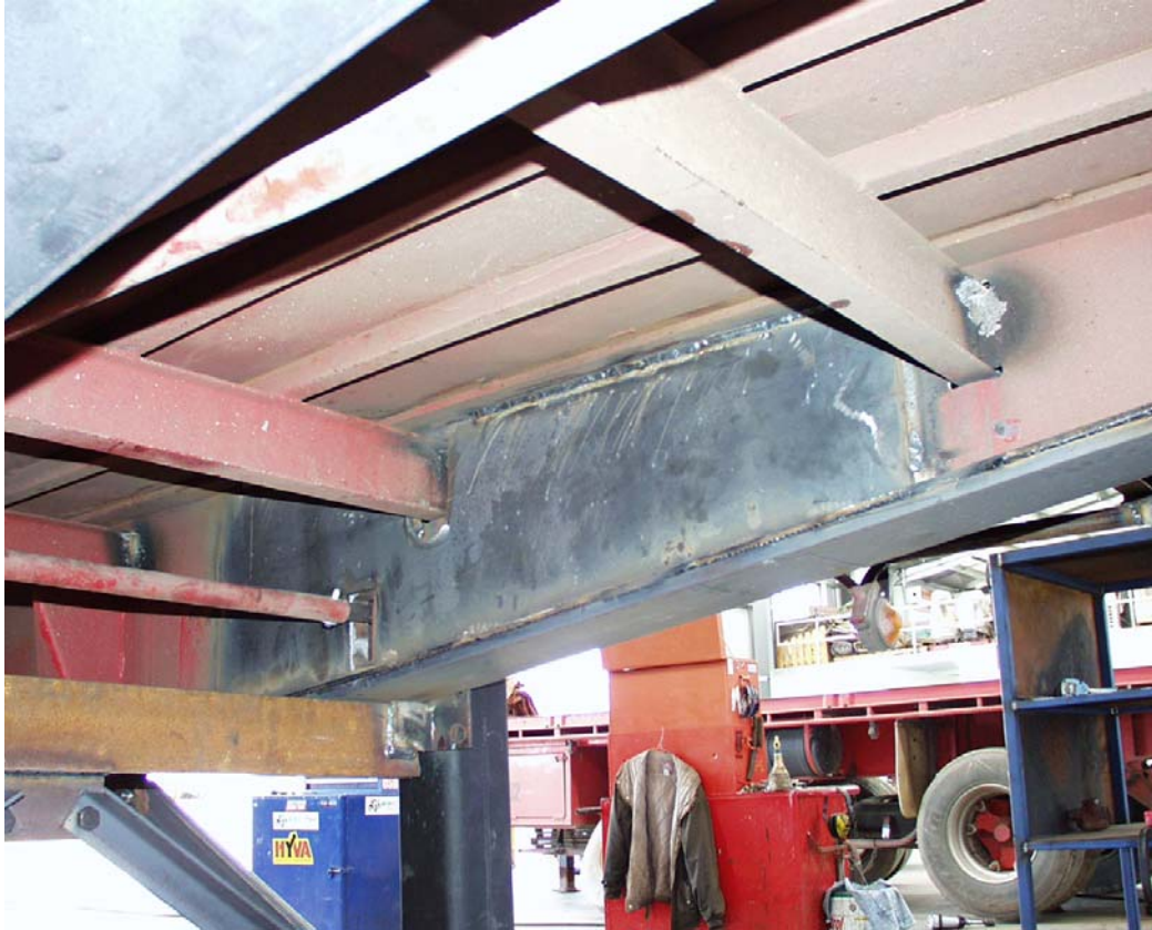
Figure 4.1 Repairs Made to Failed Neck of Flat Bed Trailer
