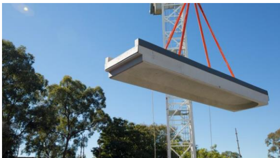
Figure 4.11: 10.8 metre geopolymer beam with vaulted soffit being craned into position Source: Aldred and Day (2012)
