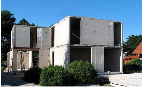
Figure 4.3: Upcycled prefabricated concrete walls – the prefabricated concrete walls of an eleven-story Stalin-era apartment buildings were upcycled into two-story villas Source: High Concrete Group (2014).
