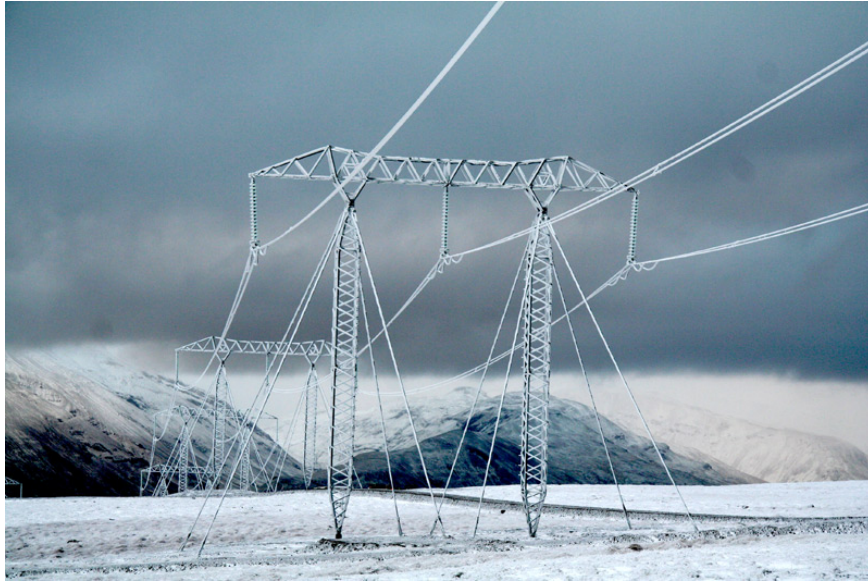
Figure 1.2: Photograph of power transmission line and structure with ice deposits. (Photo courtesy of the Landsnet (Transmission lines).)
