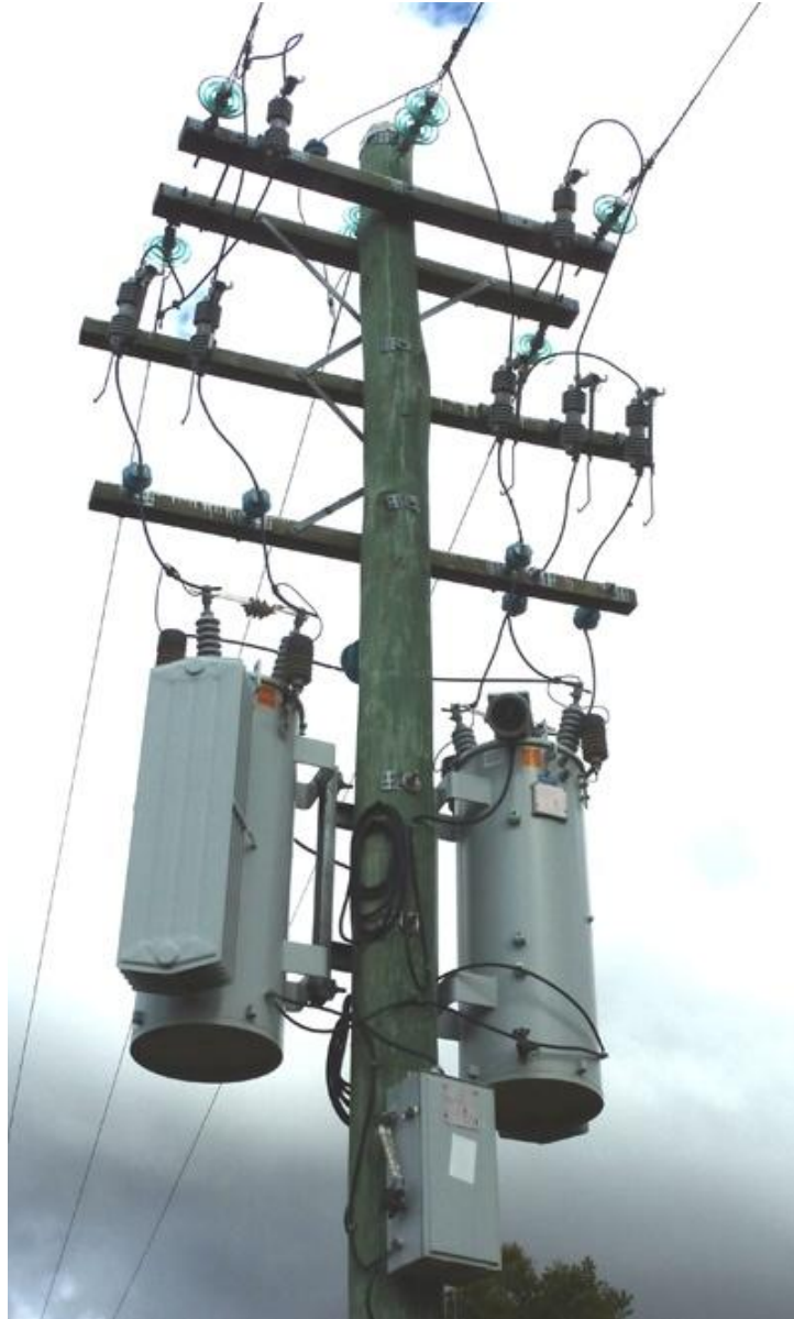
Figure 5.2 Pole mounted open-delta regulator.
