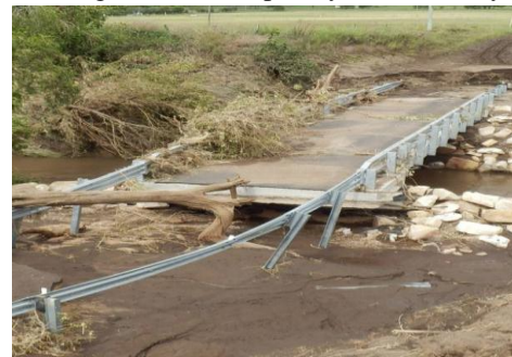
Bridge No.1 with damaged relieving slab
