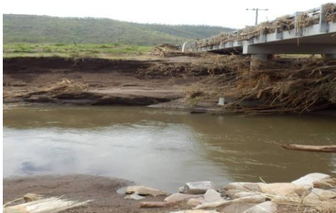
Bridge No. 2 abutment headstock damaged
