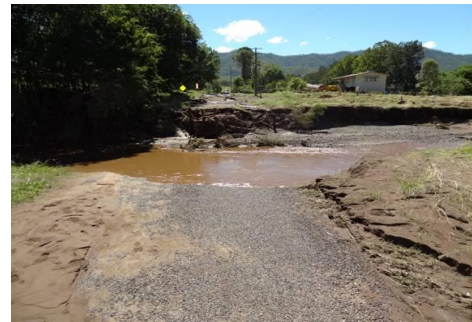
Bridge No. 16 completely washed away
