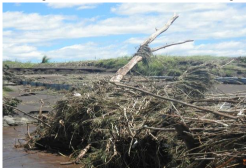
Bridge No. 8 damaged due to debris
