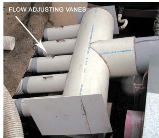
Figure 8. Manifold joining 5 individual ducts with vanes to equalise flows
