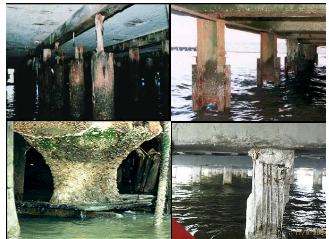
Figure 1. Degradation of traditional piles [3 & 4].
