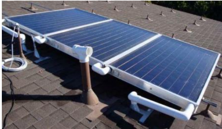
Figure 2: A sample FPC installation (Source: HubPages 2010)
