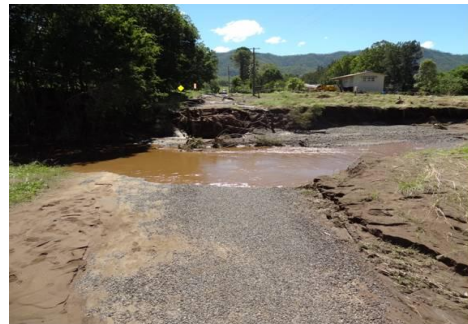
Bridge No. 16 completely washed away
