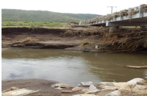
Bridge No. 2 abutment headstock damaged
