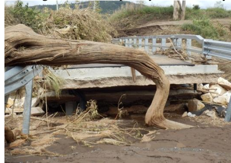
Damaged relieving slab
