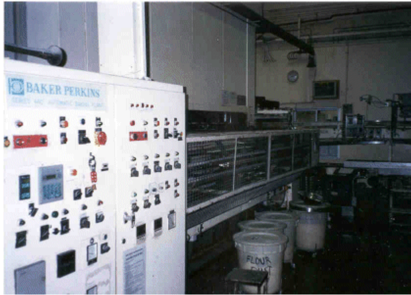
Figure B.9: Prover/Oven control panel with prover in background
