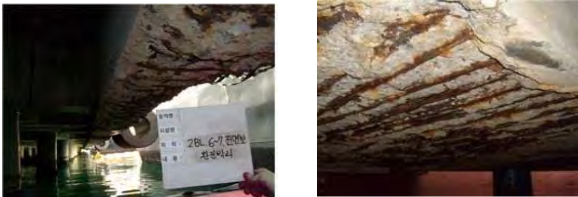
Figure 1.1 Corrosion problems of concrete structures
