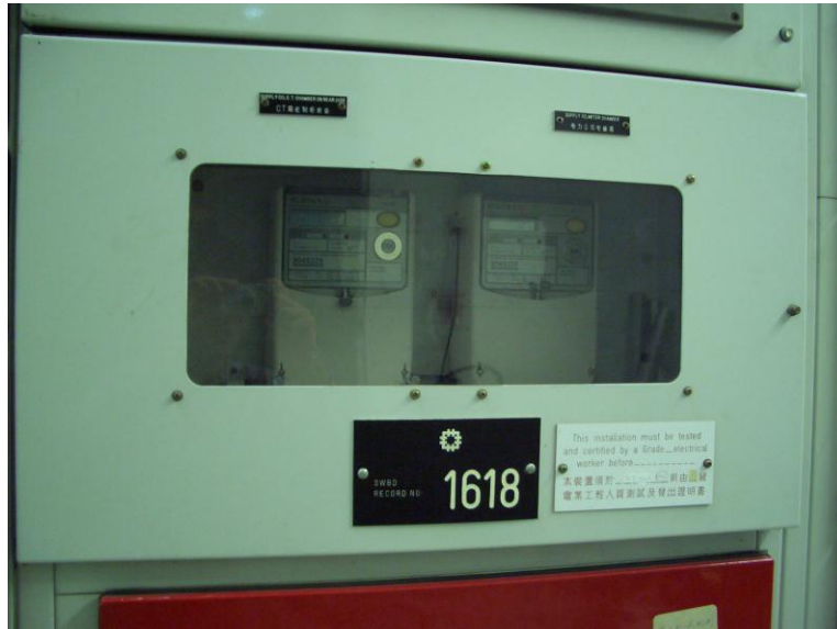
Figure 3-6 – Electricity meters in a secure rack
