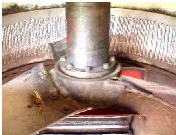
Figure 5.3: Fan assembly inside extraction chamber
