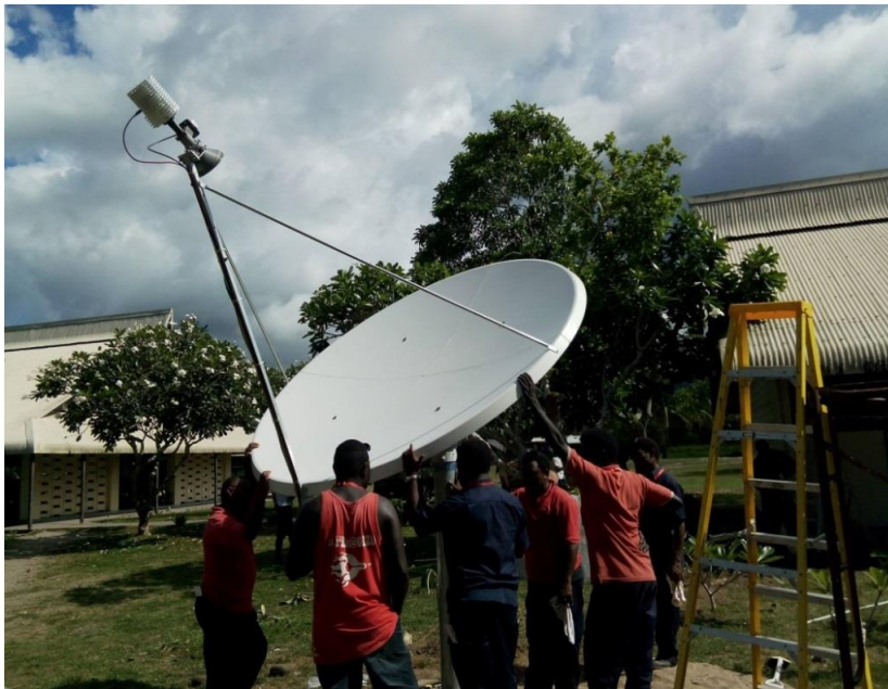
Figure 7.1 The Internet satellite dish: Solomon Telekom installed a satellite dish for the Internet at Highway NSS
