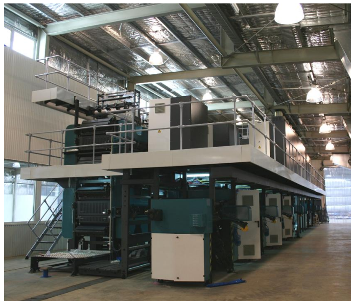
Figure 1.3 The Manugraph Cityline Express newspaper printing press – during installation at Industrial Avenue Wilsonton, Toowoomba in February 2008. Photograph – Deborah Beaumont.
