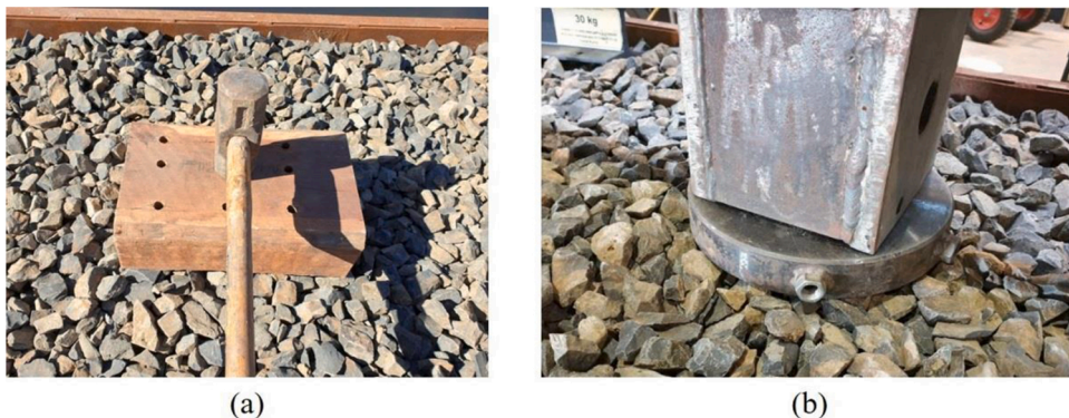
Fig. 4. (a) Ballast tamping using a sledgehammer; (b) Plate load test on the ballast.
