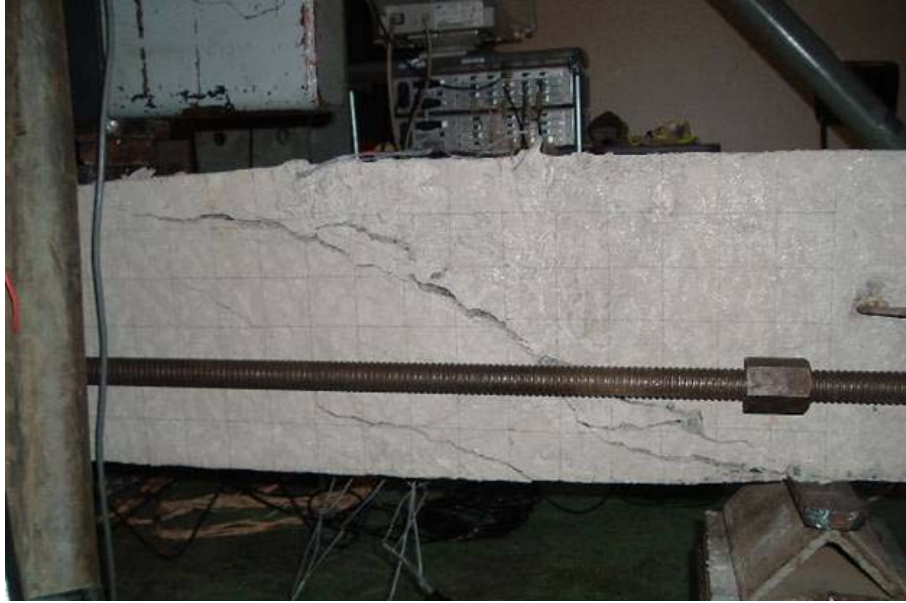
Figure 4.8. Failure of EPT12 (Post-tensioned without crack repair)
