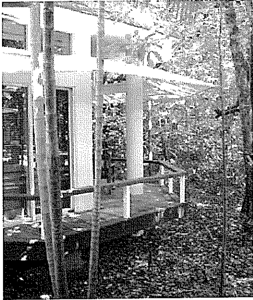
Figure 5: Elevated building with no roof gutters, Green Island Resort
