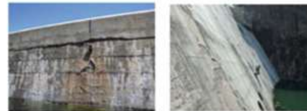
Deterioration on dam face
