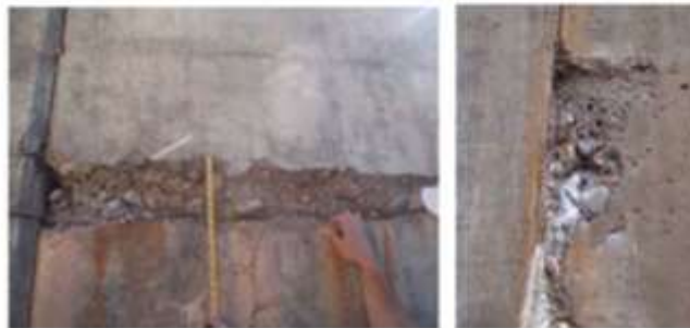
Spalling Vertical Contraction joint
