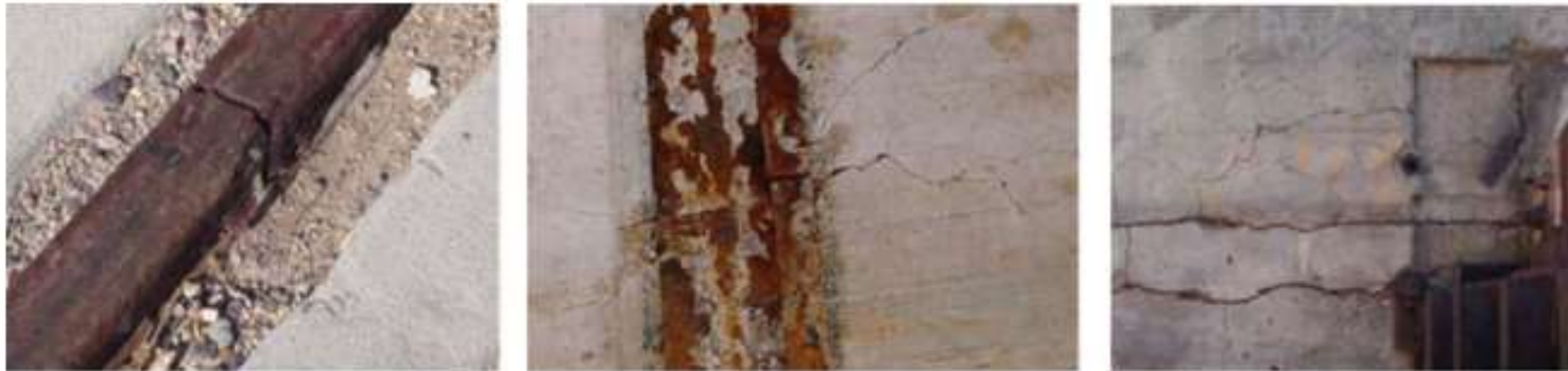
Damage to embedded mechanical equipment
