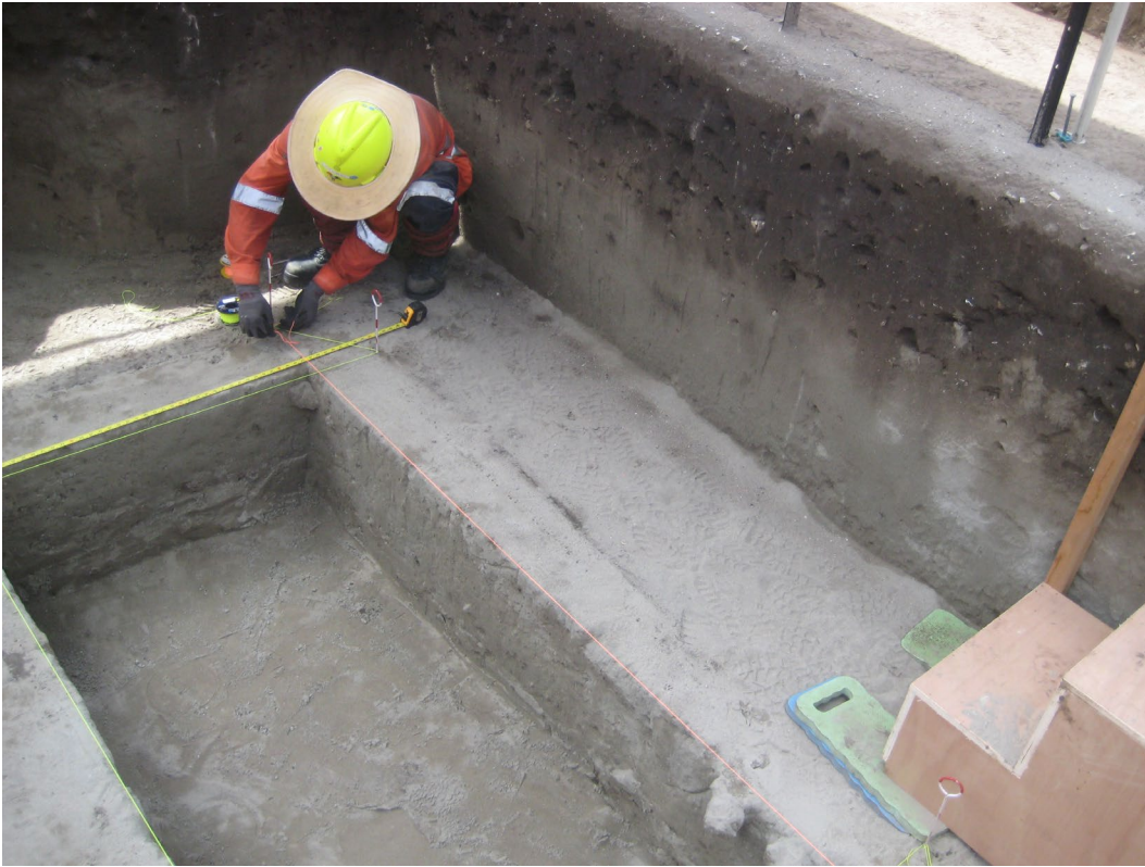
Figure 2.12. Re-stringing Squares A and B to continue excavation after removal of shoring of the outer stepping-out squares, Tanamu 1.
