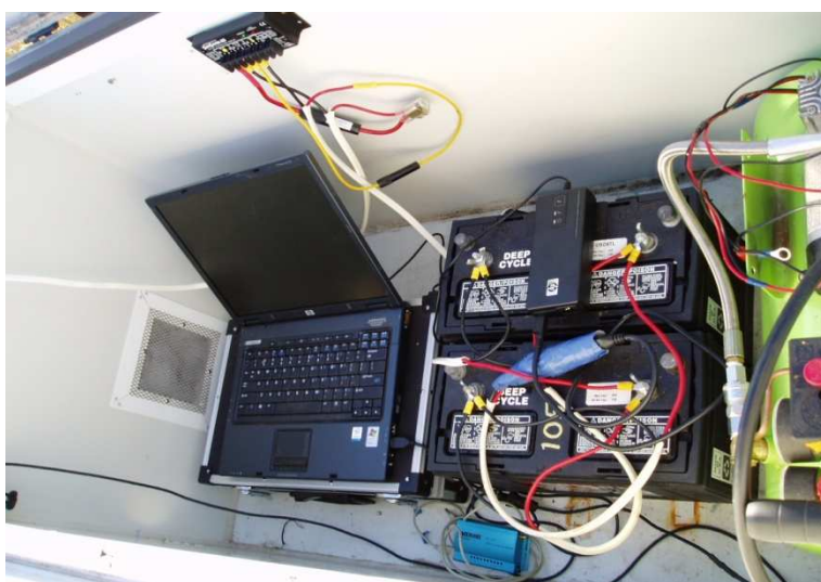
Figure 60 Laptop platform showing HP nx6120 notebook plus 2 deep cycle batteries and compressor to operate the gate.
