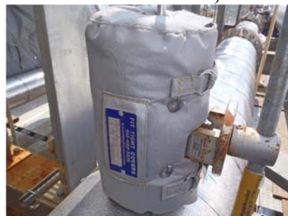
(c) Thermal shipping vessel valve insulator
