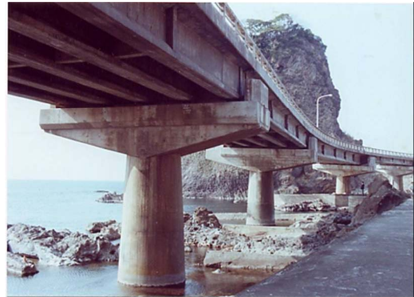
Rust and damage in girders (Kuretsubo Bridge)
