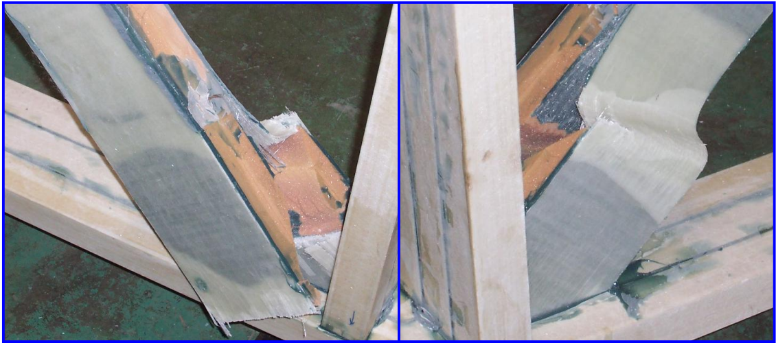
Figure 4.35 P409 - Failure at the lower corner
