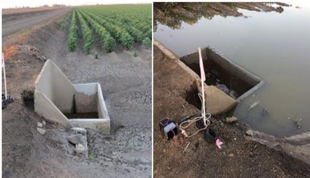
Figure 6.7 Starflow mounted on a bracket next to the concrete structure of the tail drain box at the bottom of Field 2.
