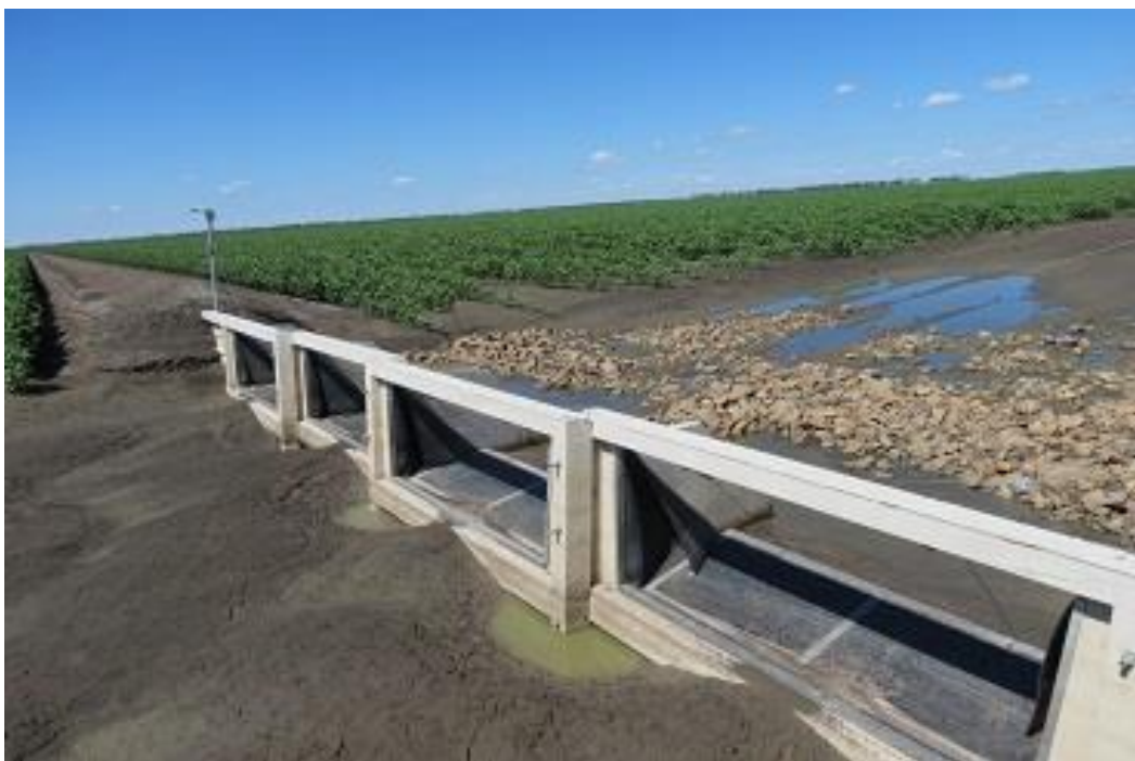
Figure 4.5 Check gate at the top of Field 2 (Padman Stops type - multi linked Padman box culverts).
