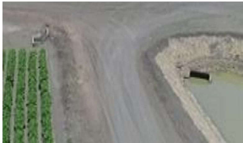
Figure 4.17 Pipe that extends underground from the tail drain box, which is located at the downstream end of the bottom of Field 2.
