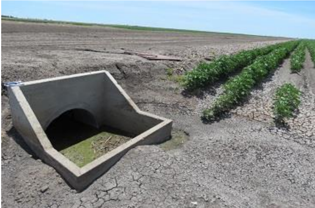
Figure 4.16 Tail drain box at the downstream end of the bottom of Field 3.
