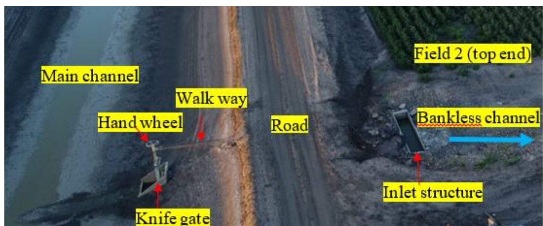
Figure 4.7 Inlet structure at Field 2, and knife gate at the top of Field 2 (includes walk way and hand wheel mounted in the main channel) that feed from the main channel to the water supply inlet. Photo taken in the Season 2, 2018. The main channel was empty.
