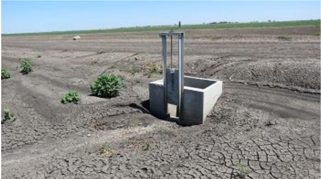
Figure 4.14 Gated drain box at the downstream end of the top of Field 3.
