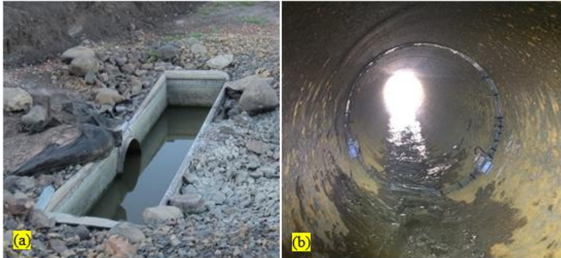
Figure 6.2 a) the inlet structure appearing at the soil surface, showing the supplying pipe 900 mm in diameter. B) Pipe ring used to mount two of Starflow in a main supplying pipe has 900 mm in diameter.
