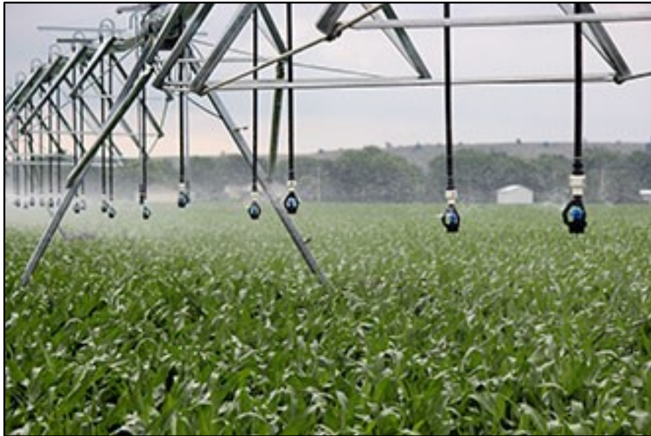
Figure 1-2: Pressure regulators installed on the upstream of sprinkler heads on a CP&LM
